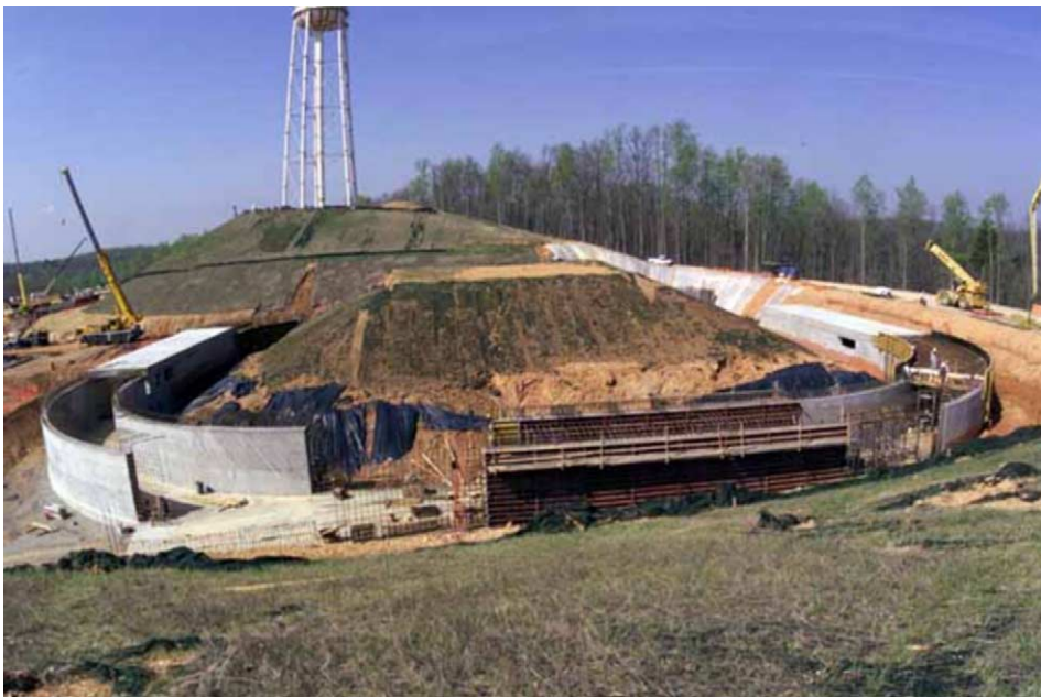
Fig. 5. Ring on side of extraction to Target Building.
