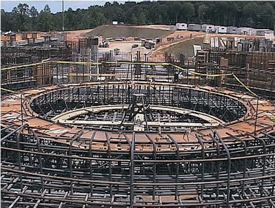
Fig. 6. Shielding monolith located in the Target Building (TB). The baseplate and lower liner will be installed soon. The liner will contain the shielding, shutter and the Hg Target System.
